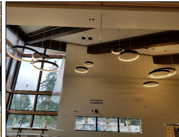
Council Chambers Lighting
